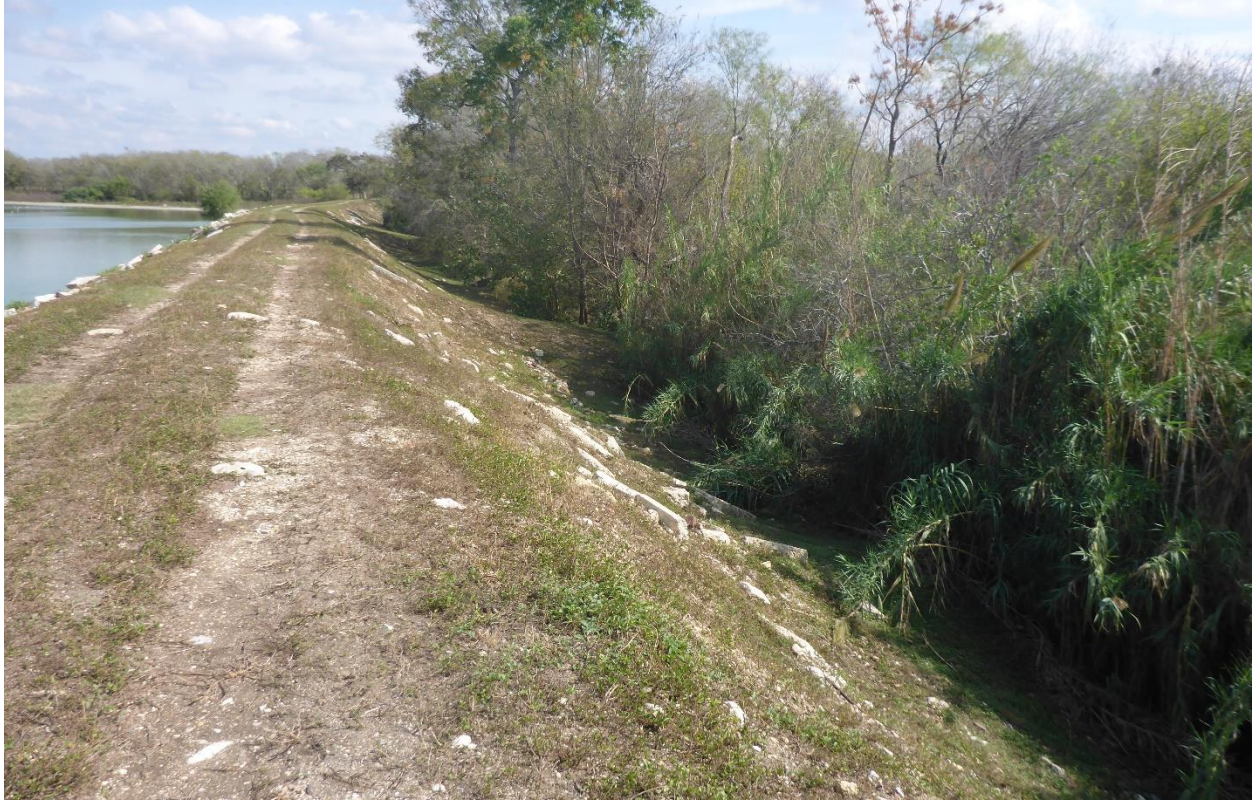
Photo 7: Downstream Embankment Slope (Note steepness and dense vegetation)
