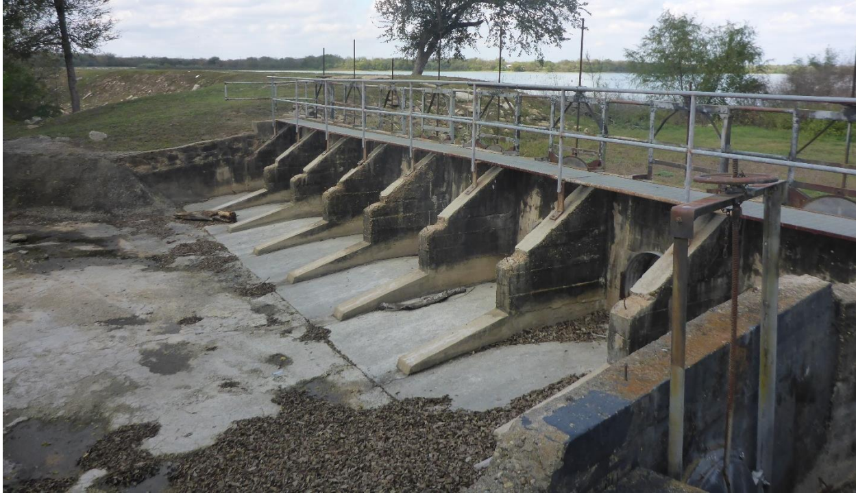
Figure 1.2: Mitchell Lake Dam Spillway (Looking Right along Downstream Side of Gate Valves)
