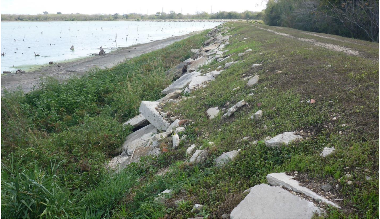
Photo 1: Embankment Upstream Face (Note steepness and sparse coverage of rubble erosion protection)
