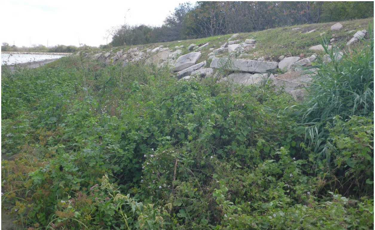
Photo 2: Dense Vegetation at Toe of Upstream Slope
