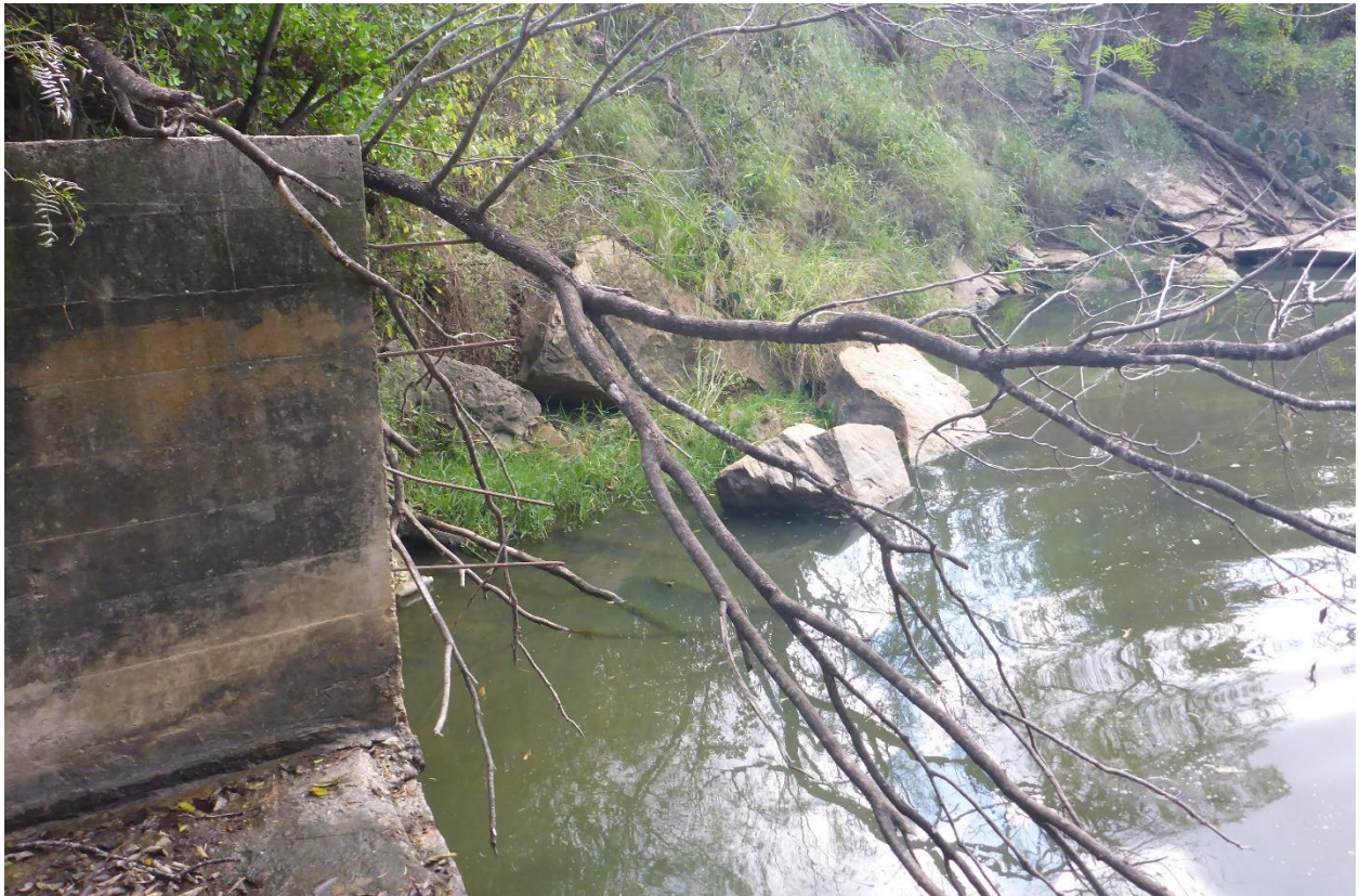
Photo 18: Spillway Channel Wall (Note exposed reinforcing steel and sheer drop)
